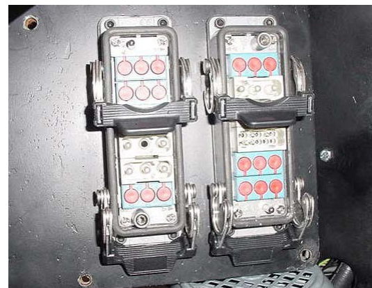
Sockets for the Inner Slip Ring Brush holder cables.
